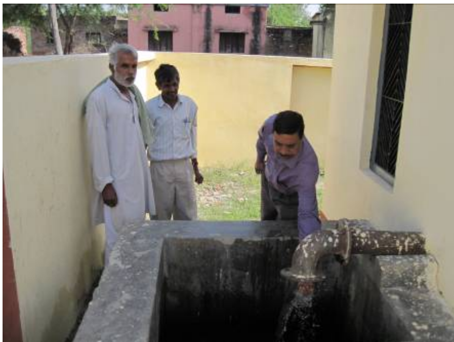
U.P. Govt. installed new water pump and appointed two staff for regular supply of water
